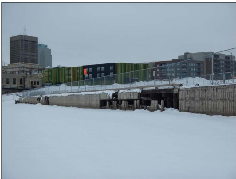
Photo 1. Photo illustrating a deteriorated section of the Alexander Dock allowing access under the dock, Feb. 15, 2017.
